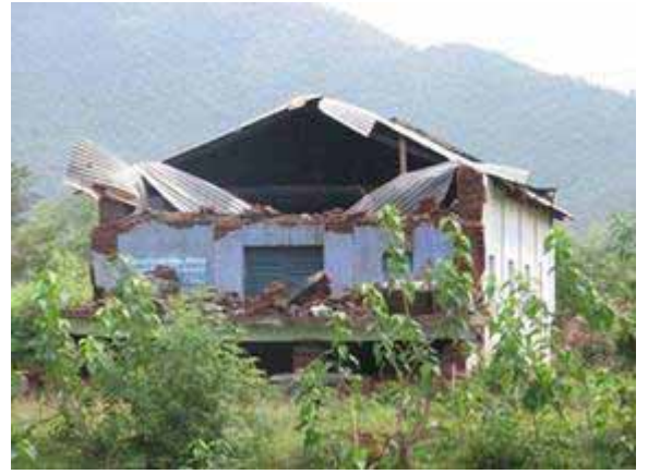
A PRAYER CHAPEL DESTROYED
